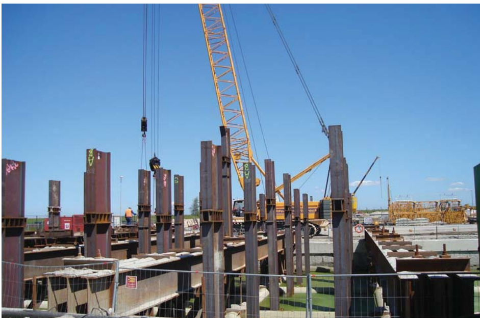
Figure 27: Use of HEB 800 with lengths ranging between 33.80 and 38.80 m as driven piles for water intake at the power plant Wilhelmshaven. During the construction phase they serve as tension piles to prevent lift, in their final function they transfer loads.
