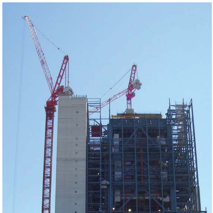
Figure 18: Boiler house of the power plant Wilhelmshaven, Germany
