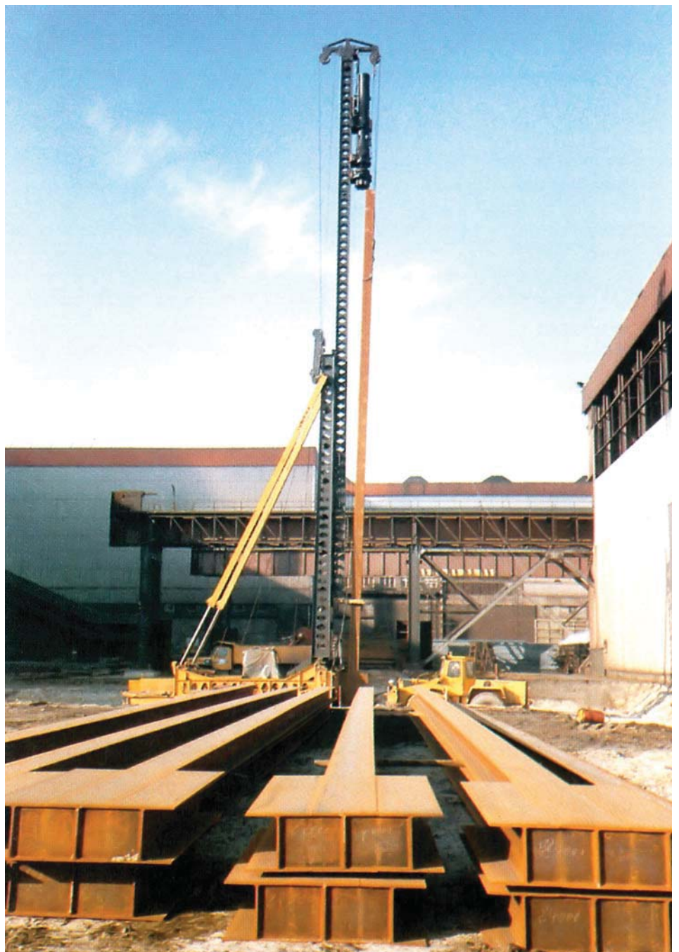
Figure 28: Driven piles with reinforcement at the base to increase the cone friction resistance and thus provide support for high loads
