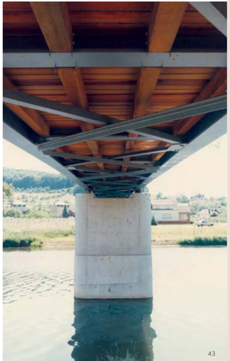
Bottom view on the stiffening elements of the bridge in Steinheim, Luxembourg
