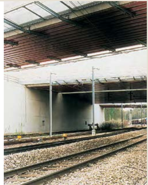
Filler beam bridge built over a heavy traffic railway line – High quality coating provides durable protection to lower flanges.
