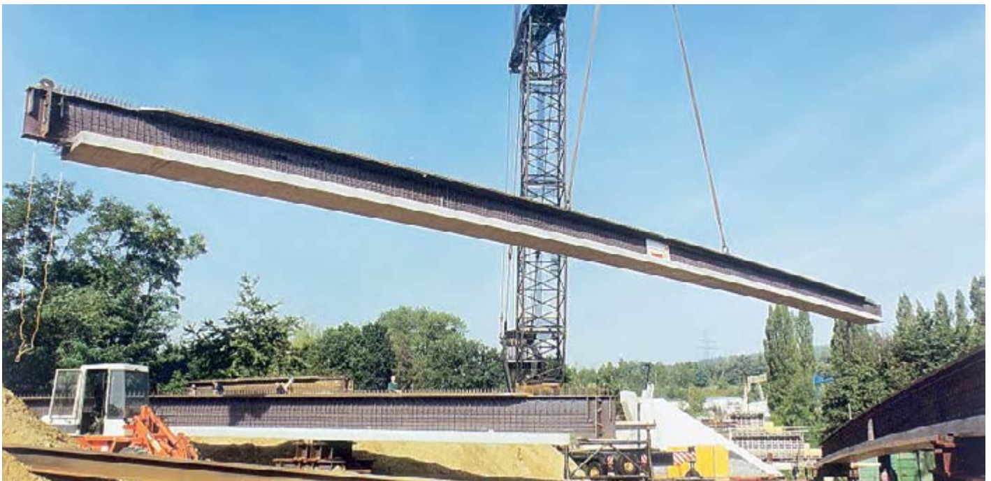
Single span bridge in Kerpen Horrem, Germany - 41.25 m long HE 1000 A beams used for prestressed composite girders of "Preflex" type.
