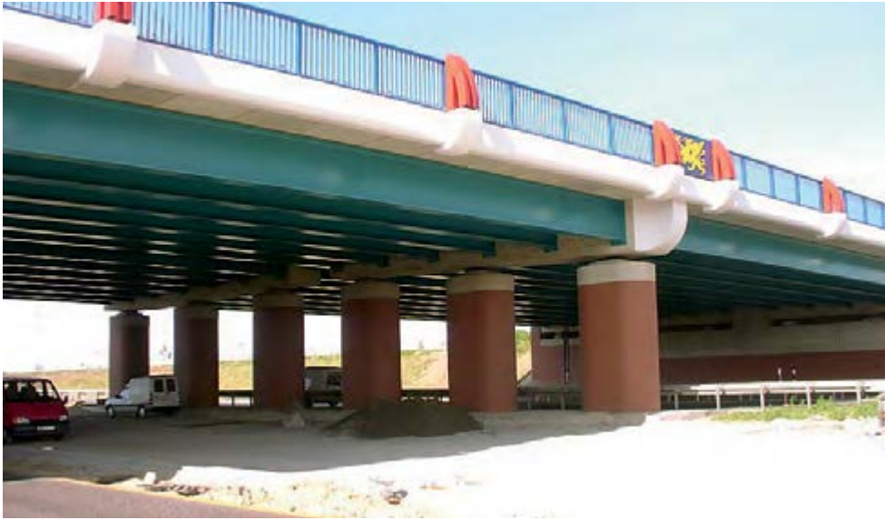
Composite bridge with concrete crossbeams at Bentwisch, Germany – Design combining steel and colour.
