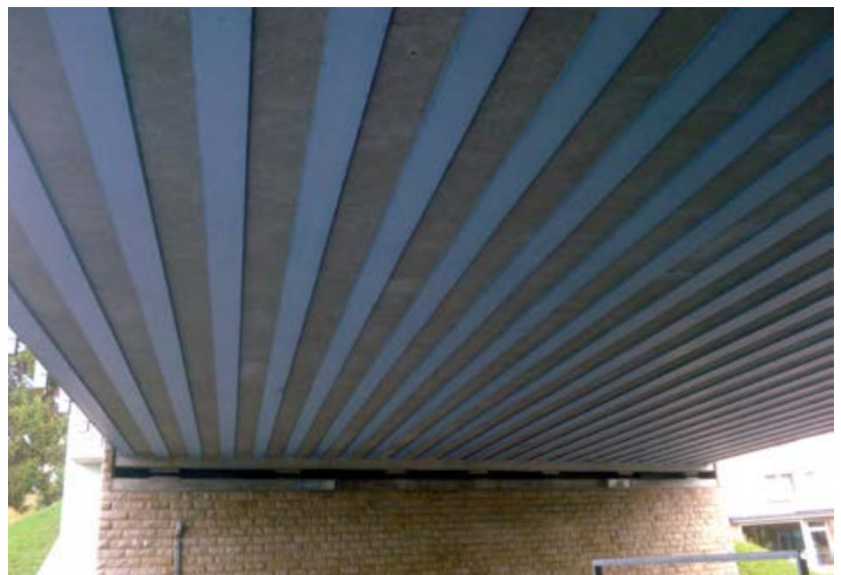
Lower side of a filler beam deck – Only the bottom flanges of beams are visible.
