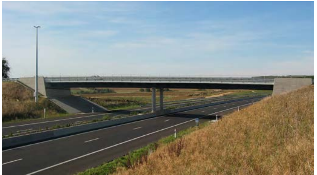
Bridge link with two spans of 23.9m to La Sarre, Luxembourg – The composite bridge is a twin-girder bridge with box sections of two longitudinally welded rolled beams.
