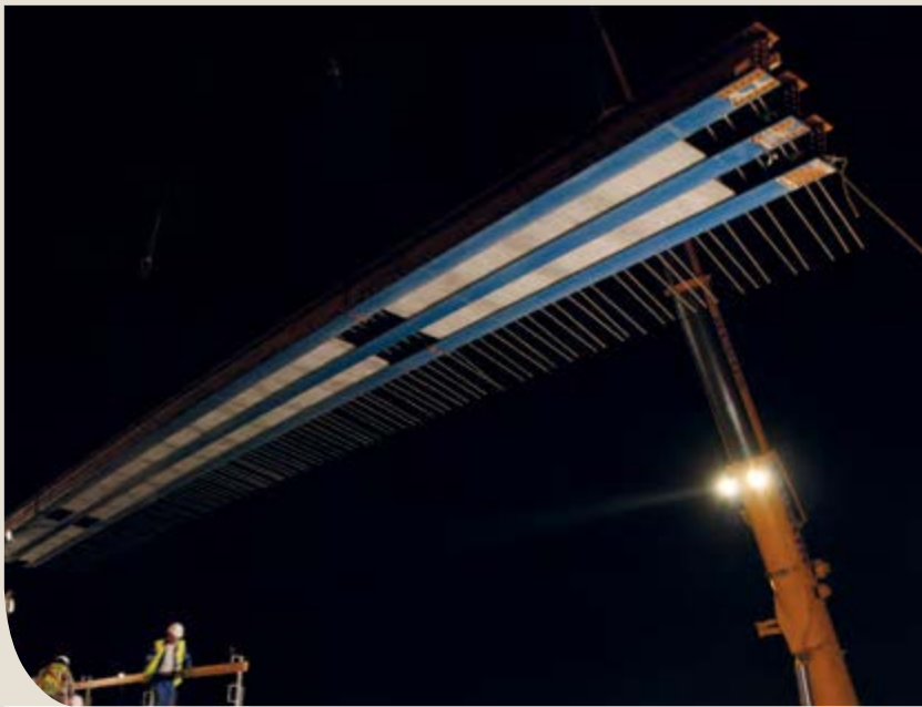
Railway bridge at Sète-Frontignan, France - Lifting in of a pre-assembled part over an existing railway line.
