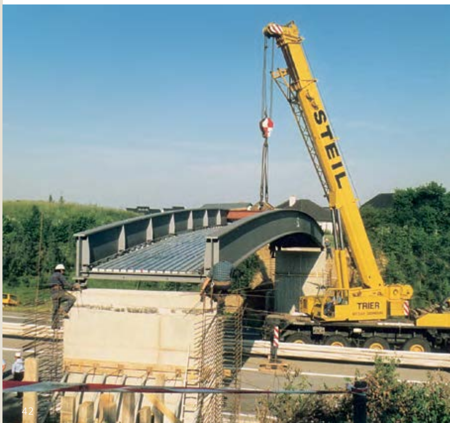
Erection of half-through type structure – Pre-assembled framework including permanent steel shuttering is lifted into position by crane.
