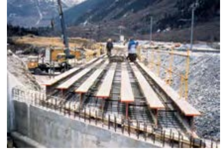
Construction of a filler beam railway bridge as part of the Puymorens road tunnel link between France and Spain.
