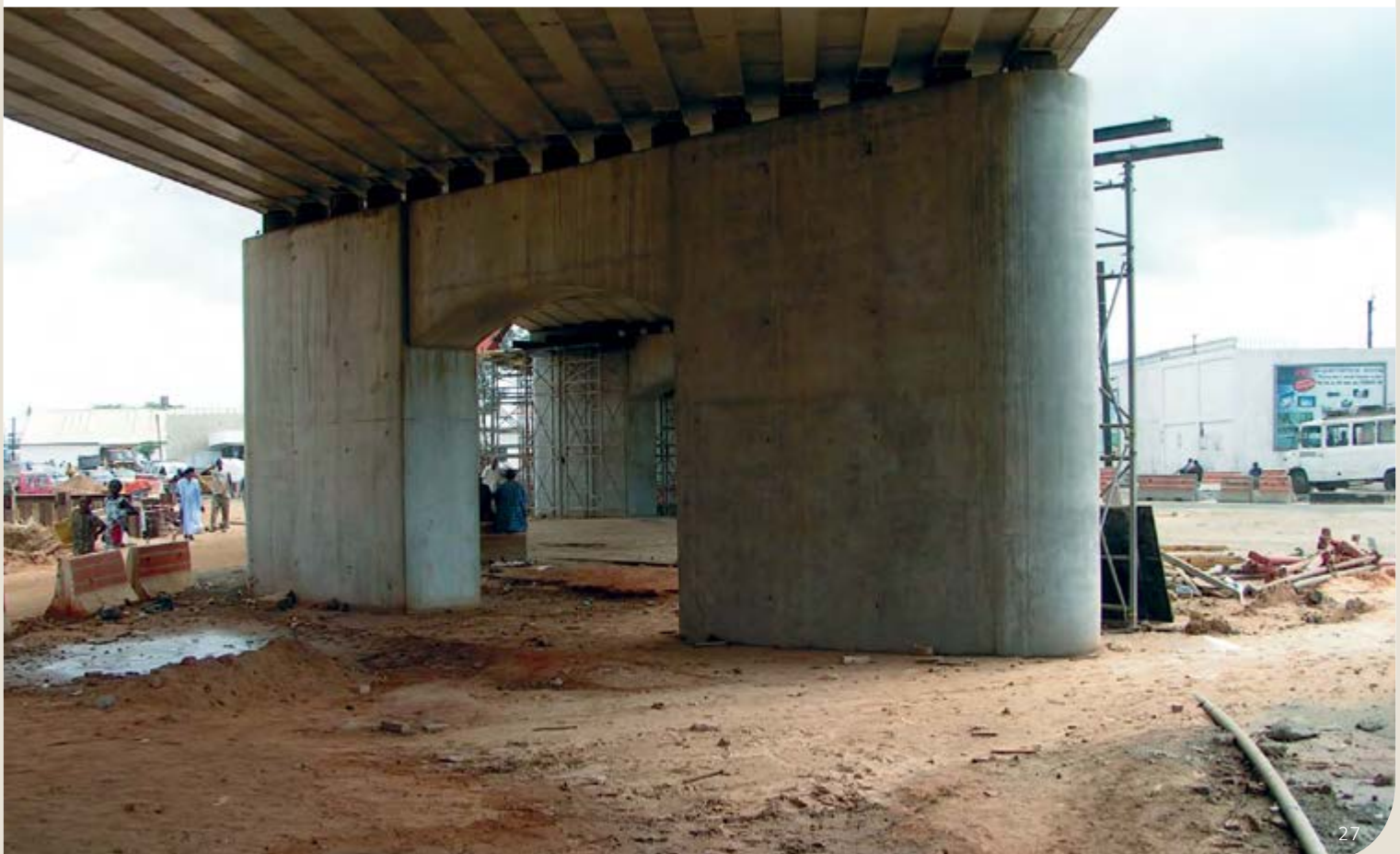
Pont de Cyrnos in Senegal - Bottom view on the filler beam deck and support.
