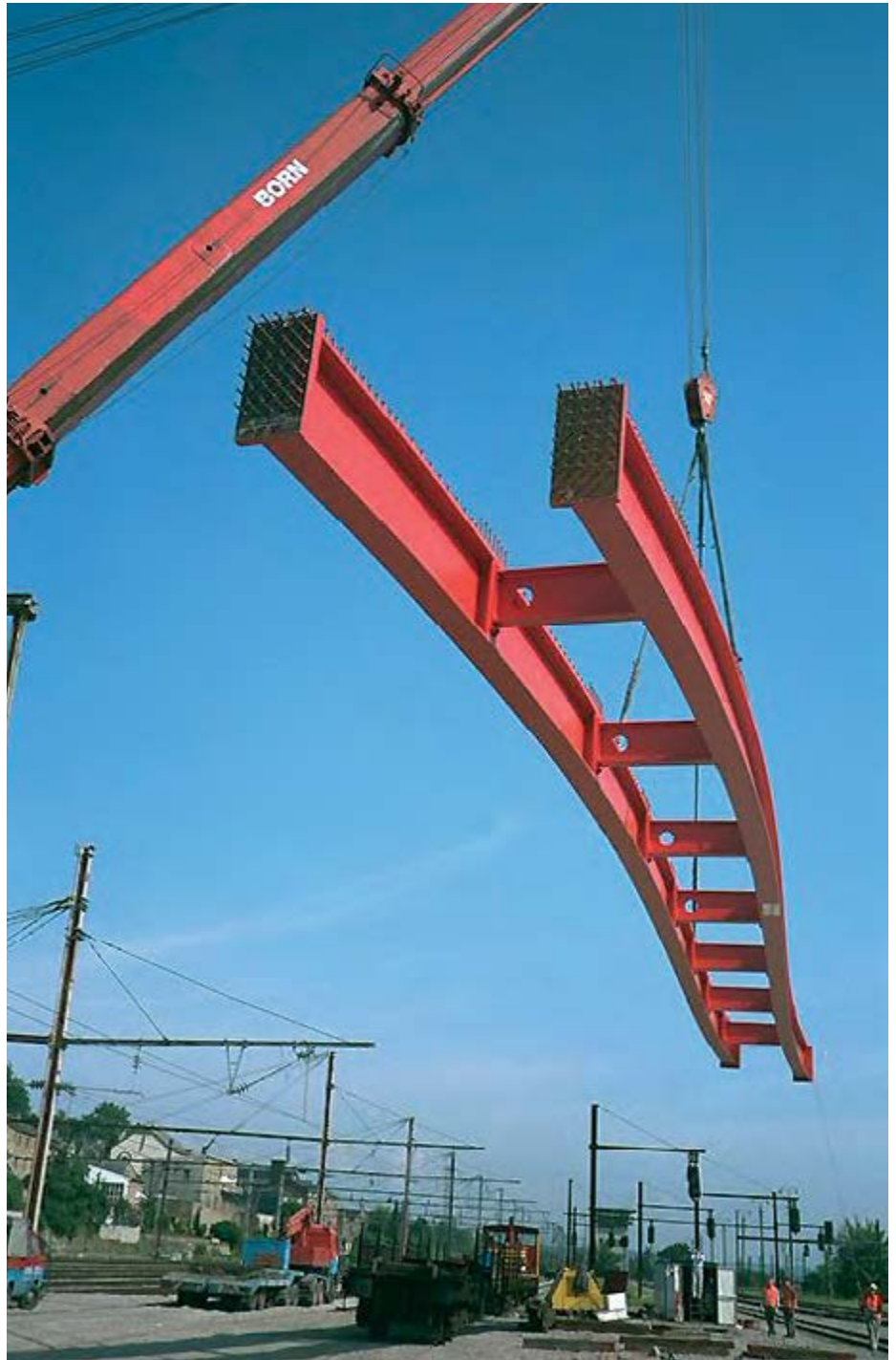
Road bridge in Differdange, Luxembourg – Erection of two main girders of a composite bridge by crane. The rolled girders are curved along both cross-sectional axes in order to adapt them to the geometry of the road.
