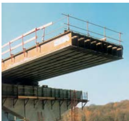
Railway bridge of the TGV Atlantique high speed line in Massy, France – Launching of the beams over the A10 motorway interchange.
