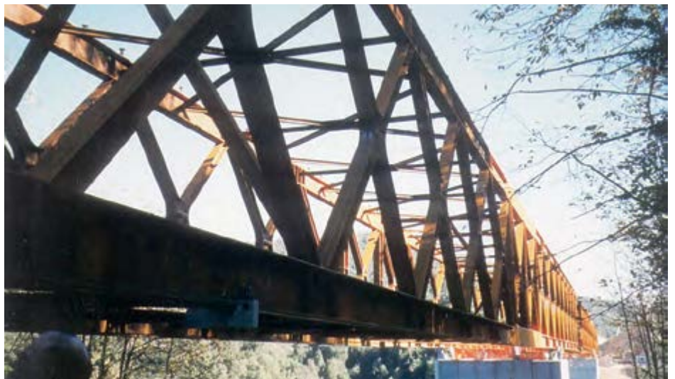
Costa Martina road bridge, Spain - Rolled beam truss girders, continuous over 3 spans of 60.6 - 121.2 - 60.6 m. The picture shows the bridge before the erection of the precast slab elements on the upper chords.
