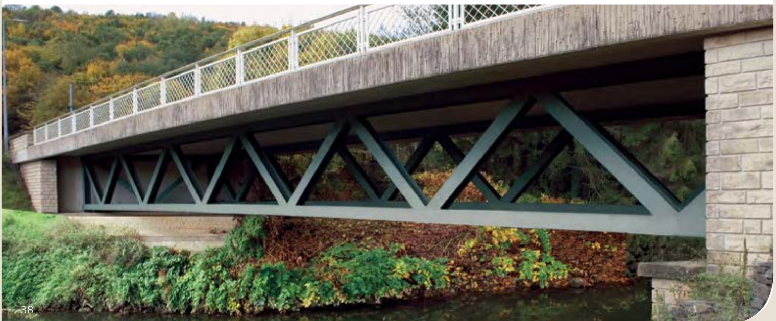
Bridge over the Alzette river in Cruchten, Luxembourg – Transparent truss structure in composite action without gusset plates – S460 rolled steel sections have been used as truss members.
