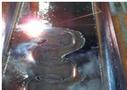
Oxycutting of a rolled beam (HD 320x300 in S460) with MCL shape for a PreCoBeam bridge in Germany.
