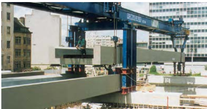
Extension of the Brussels - South Station for the Eurostar trains - A launching gantry is used for fast erection of prefabricated prestressed composite decks.
