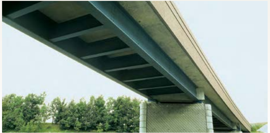
Railway bridge over the A23 motorway in Fretin, France – Four-span bridge with spans of 16.9 – 21.9 – 23.0 – 17.8 meters. The two continuous main girders and the bracings within spans are rolled beams; the cross beams at supports are made of reinforced concrete.
