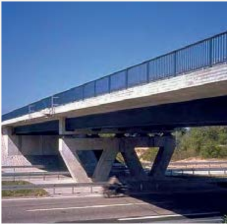
Road bridge in Bremgarten, Germany – With concrete cross beams and indirect support.
