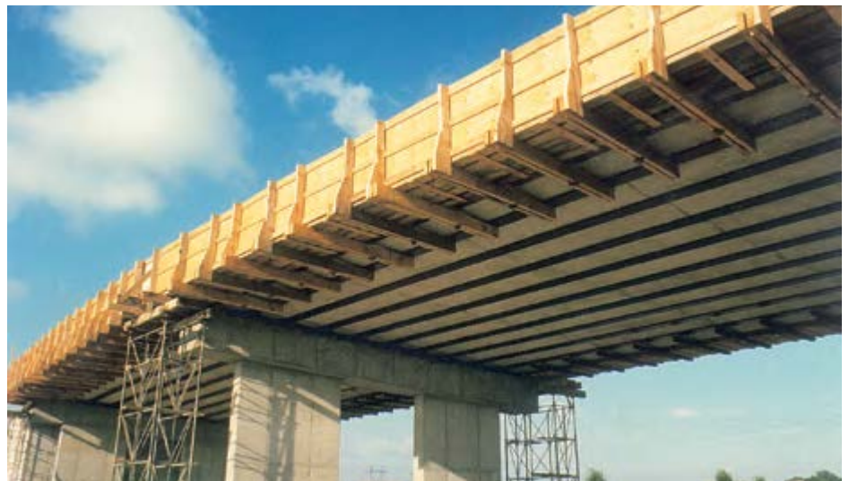
Construction of an overbridge of A104 motorway, France – Falsework is not required. Disruption of motorway traffic is minimal.
