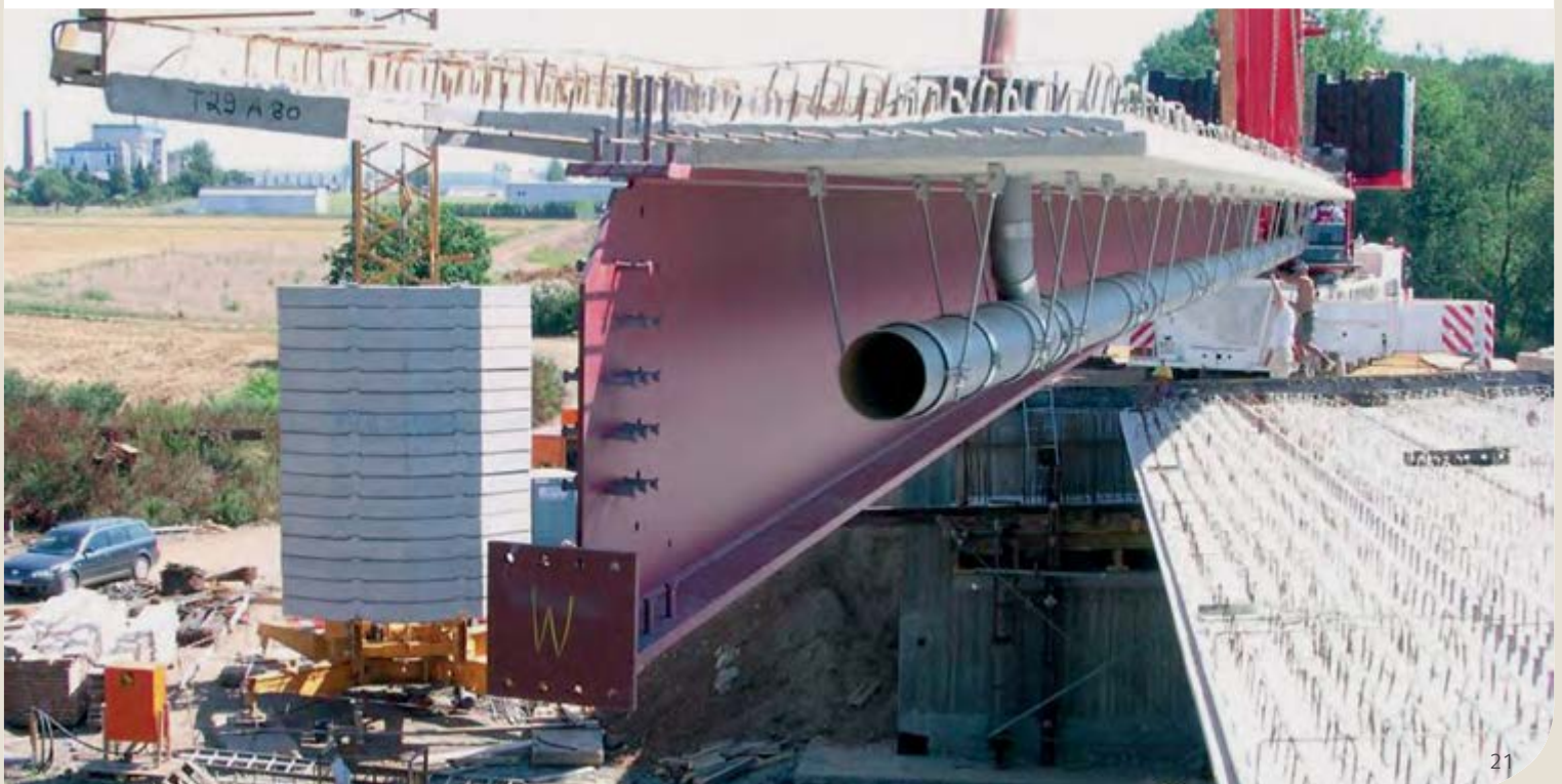
The Horlofftalbridge in Hungen, Germany - Lifting in of a partially prefabricated beam.
