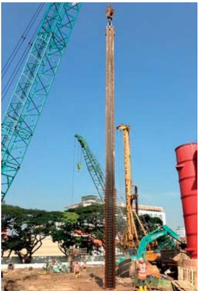
Figure 8.3: 26-metre long foundations for the top down construction method with no splicing required.
