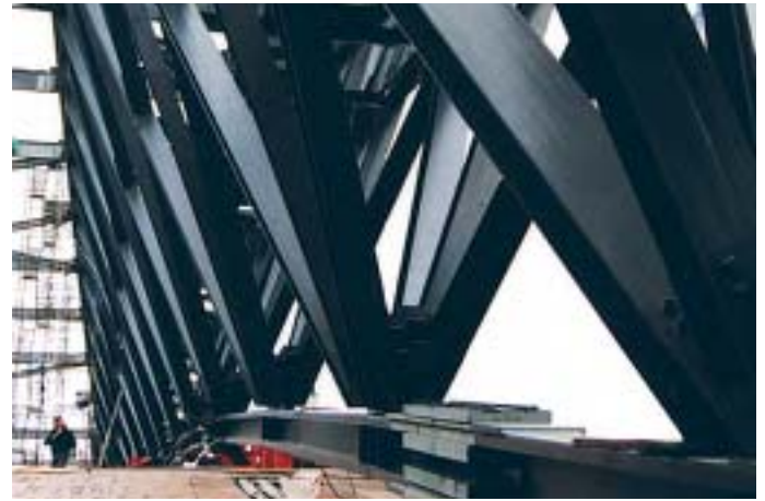
Figure 7.5: Gusset plates connection in S355 (Gr .50) with S460 (Gr. 65) beams at Mariner Stadium (Seattle)
