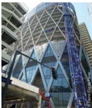
Figure 2.1: Tour D2, half of the weight is carried by exterior steel diagrid, Courbevoie, France
